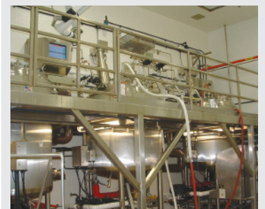
Stationary Vessels in Compound Room
