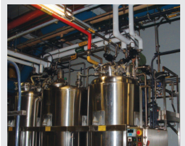
DI Water Skid in Central Utility Building
