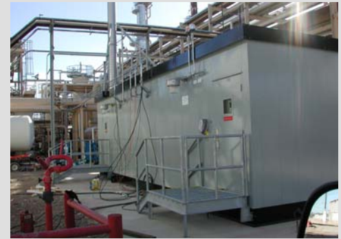
Remote Instrument Enclosure in Place
